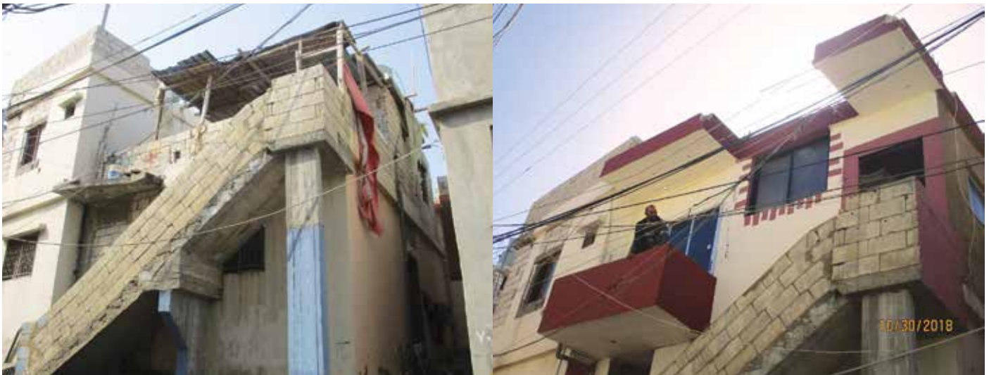
Before and after photo of a shelter rehabilitation initiative in Rashidieh refugee camp, Lebanon.
